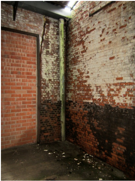
Foto 12: RWA in asbestcement in loods B
